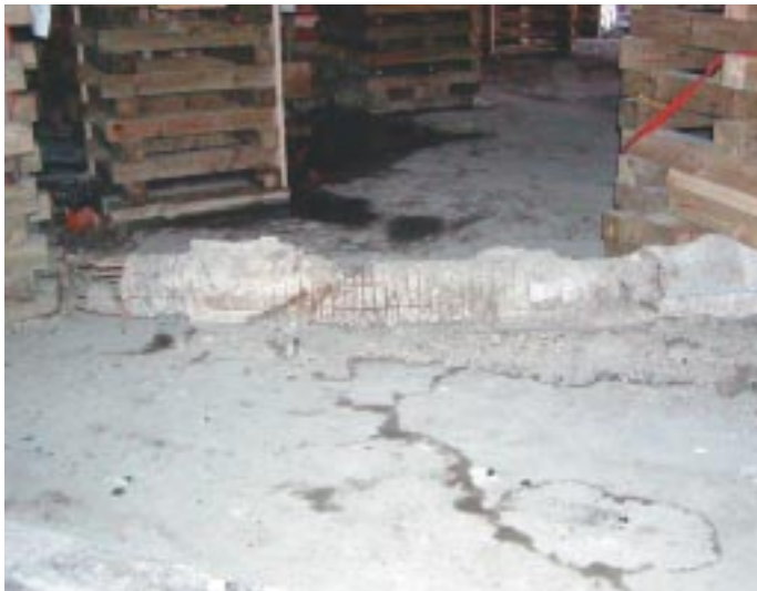
Figure 7.5a Column impacted and torn off at supports
