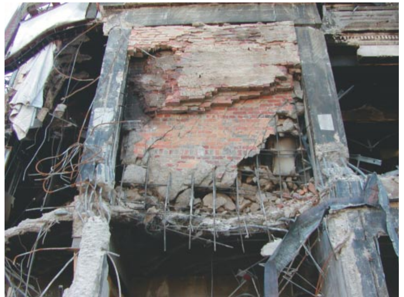
Figure 5.12 Gashes from impact of right wing
