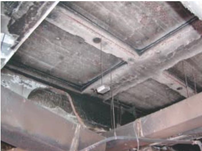
Figure 6.12 Fire damage to third-floor (light well) beams
