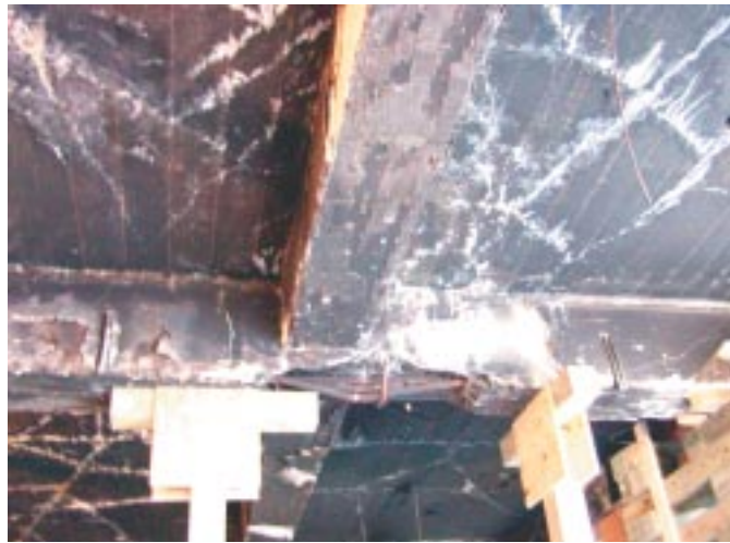
Figure 6.14 Fire-damaged second-floor beams
