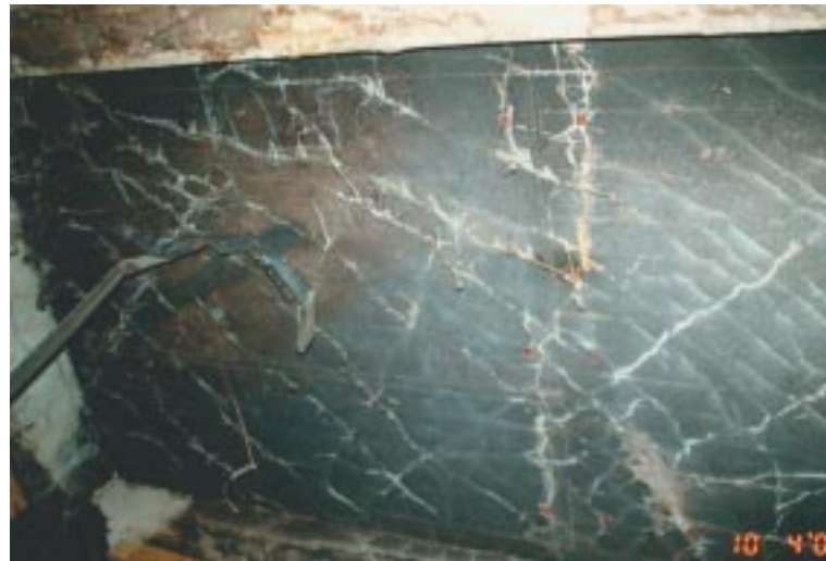
Figure 5.28 Crack patterns in second-floor slab
