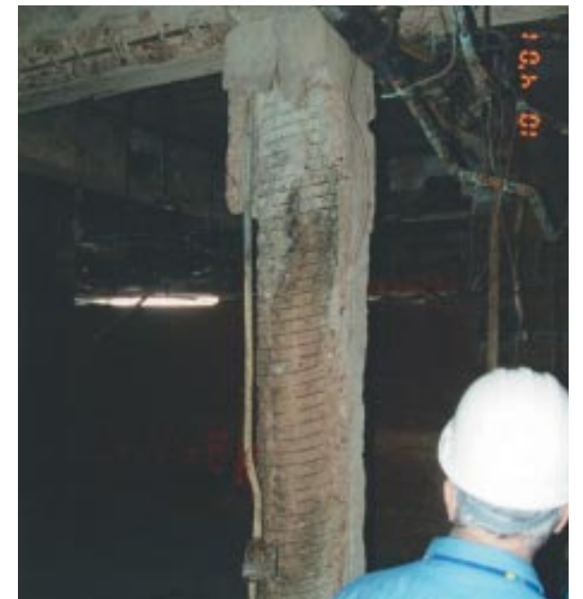
Figure 5.31 Fire damage to column in second story
