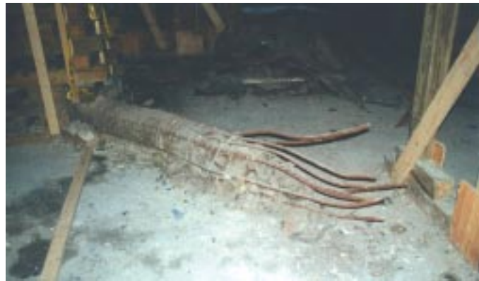
Figure 5.23 Severed column 5H
