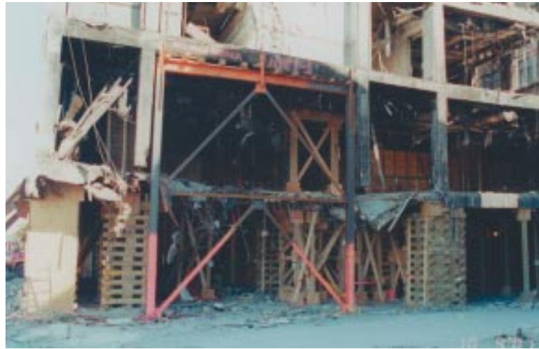
Figure 5.5 Missing first-floor columns 11A, 11B, and 11C
