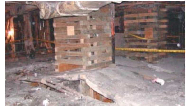
Figure 5.27 Breached second-floor slab
