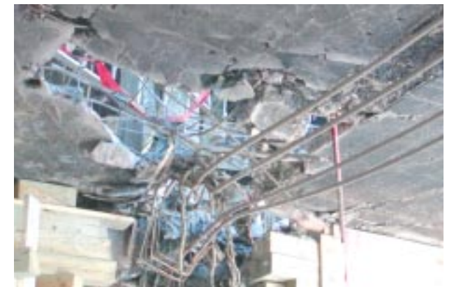
Figure 5.29 Concrete stripped from floor beam
