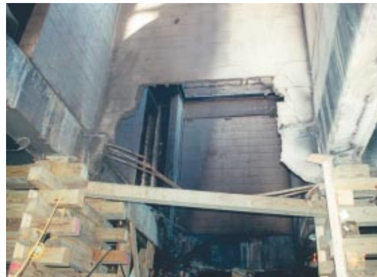
Figure 5.30 Missing beam in air shaft
