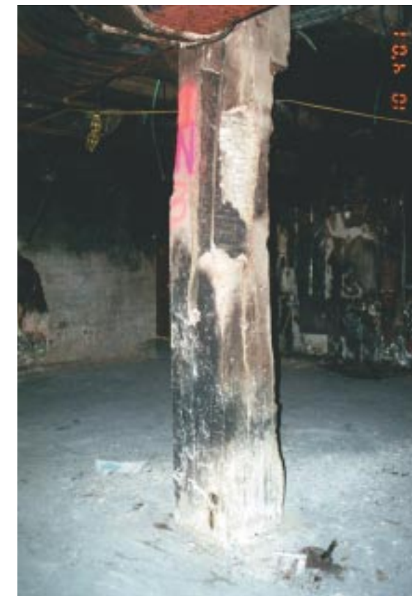
Figure 5.19 Column 3N damaged by impact and fire
