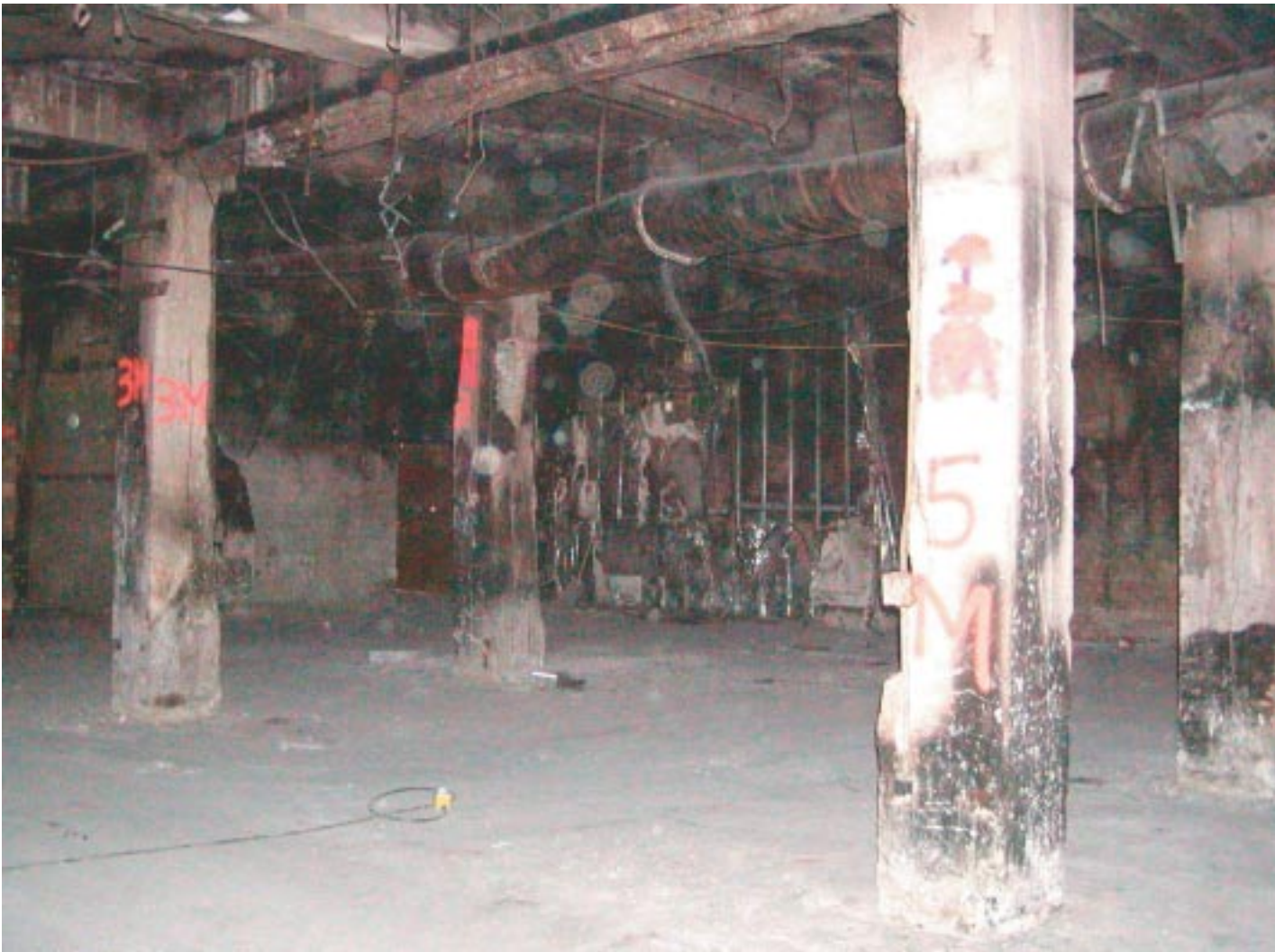
Figure 6.8 First-story columns 5N and 5M
