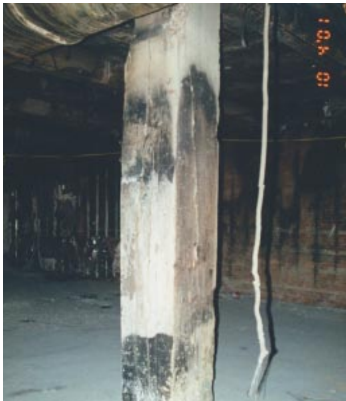
Figure 5.24 Cracked column 5N
