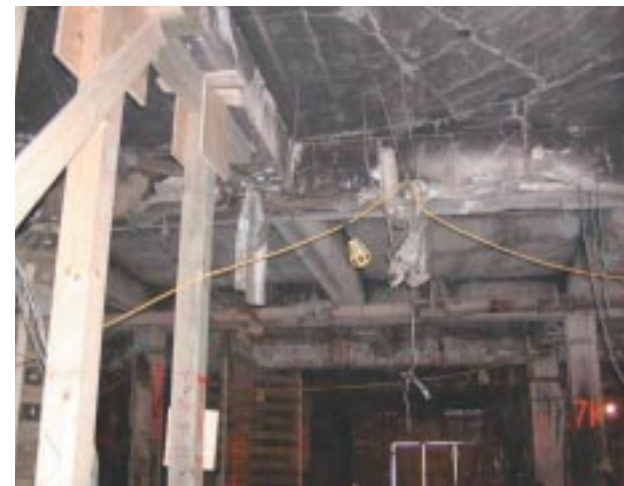
Figure 5.26 Impact damage near column 6K
